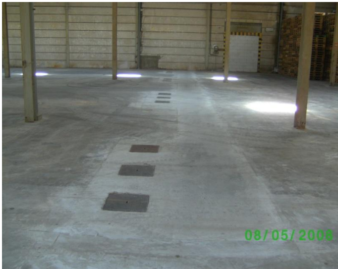
Figure 3. Pictures of the installation
