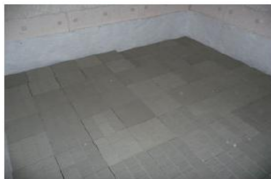
New packing type (honeycomb) installed in Thermal Oxidiser
