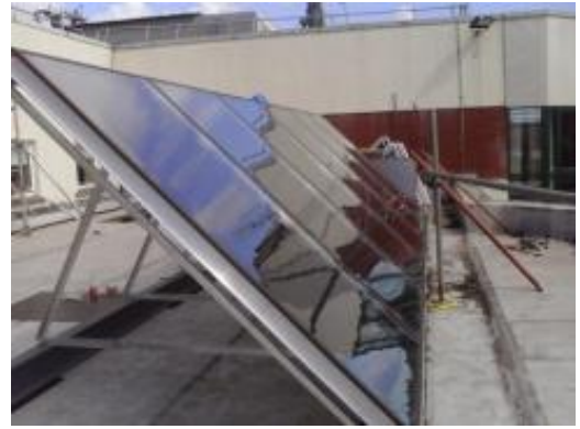
Solar panels on the roof of the administration building
