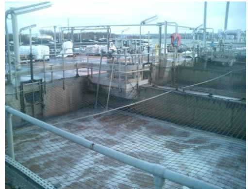
One of the aeration basins in the waste water treatment plant
